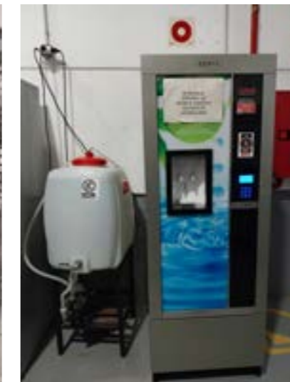
Tank collecting water from the osmosis machines
